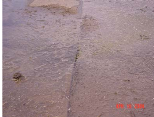
Groundwater seep between asphalt overlays
