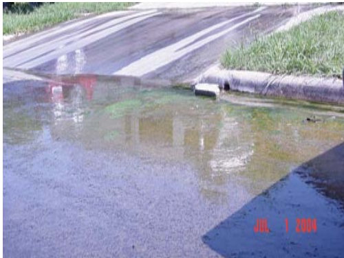
Groundwater seep piped to a curb and gutter outfall with seepage from between sidewalk and driveway.
